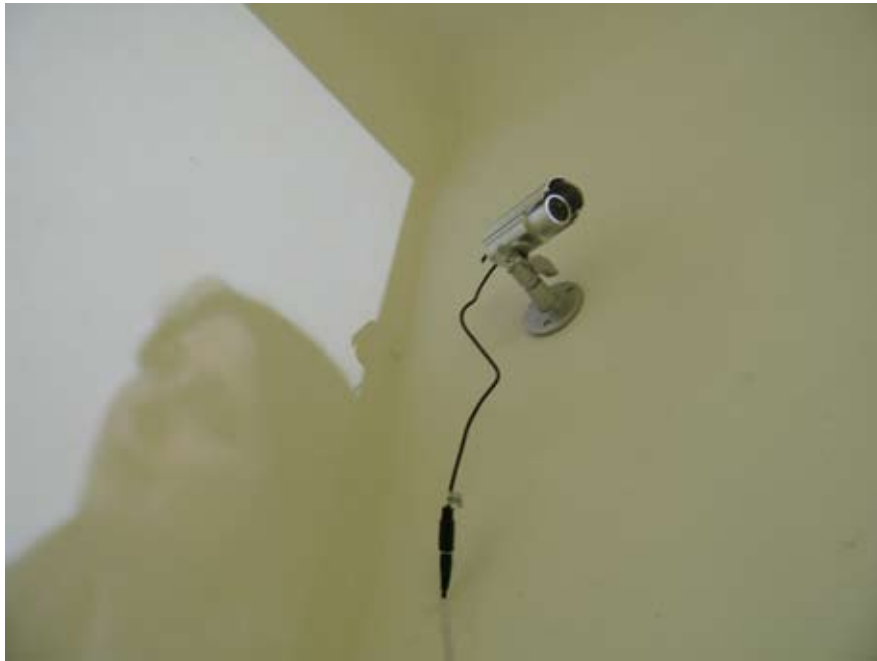
Christoph Srb installed CCTV cameras to monitor the making of the 'FUNding FACTORY'.
